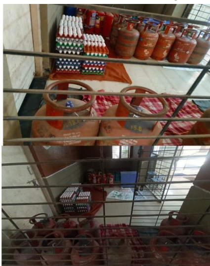
The gas cylinder and fire extinguisher and inverter battery are in the same room .
