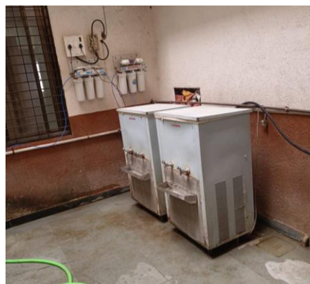
Water cooler is rusted and not in working condition
