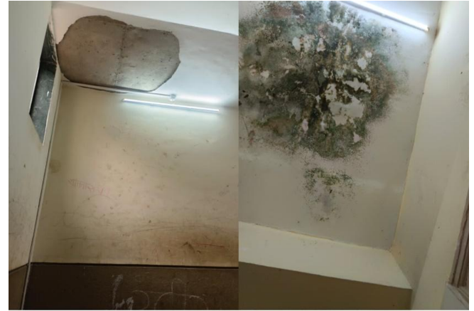
Ceiling Wall of the boys hostel
