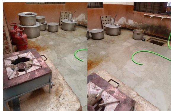
Open drainage system in the kitchen of boys hostel ashramshala
