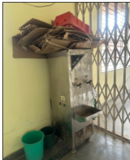
Broken water filter. There were leaves and dirt accumulated in the drinking area
